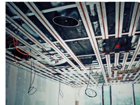
Above the suspended air-conditioning ceiling of the RBZ BIBERACH there is enough space for ventilation ducts and other elements of the building services.
