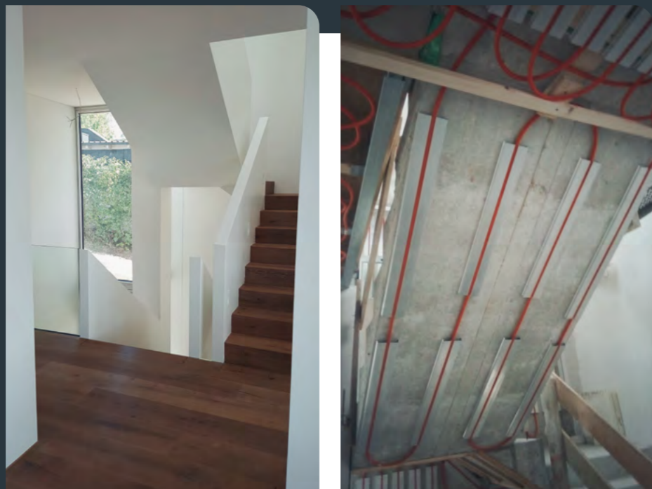
Single-family house with air-conditioned ceiling to the open stairwell.
